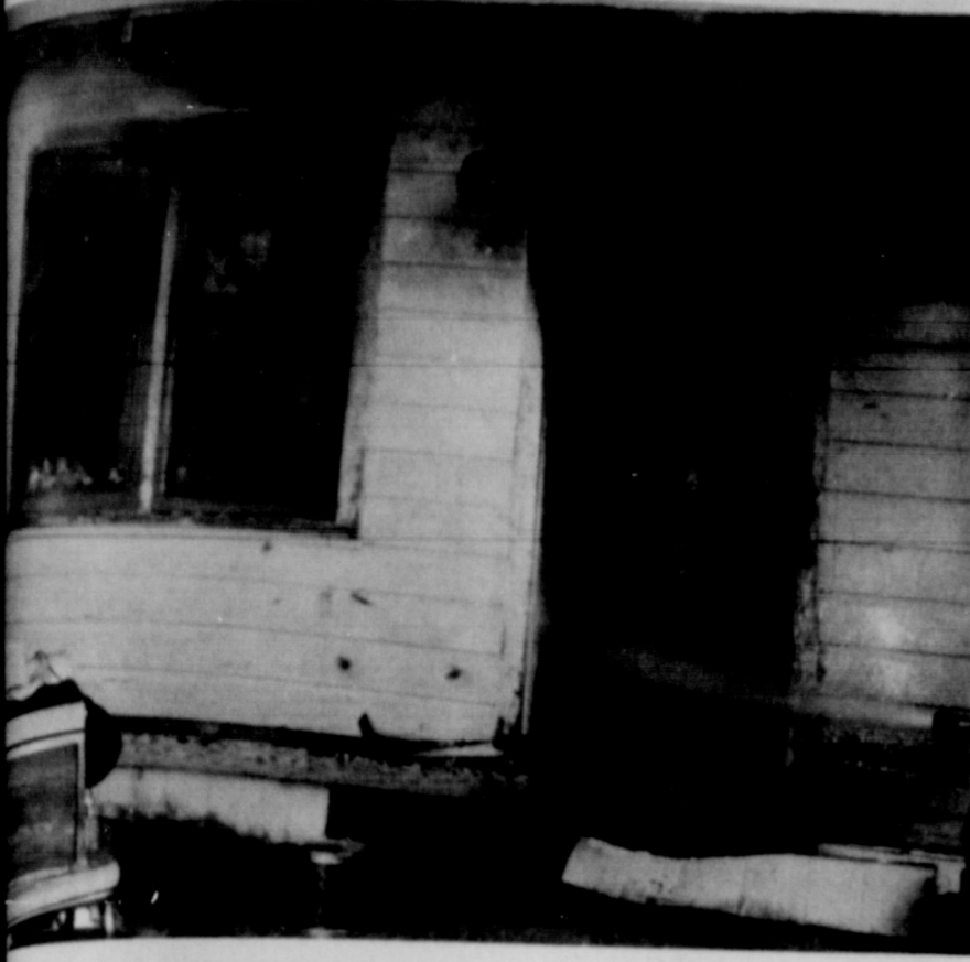
BLAZING --This photo shows that the inside of the Bob Hopper home north of Slaton is blazing. The home burned Wednesday. (SLATONITE PHOTO)
