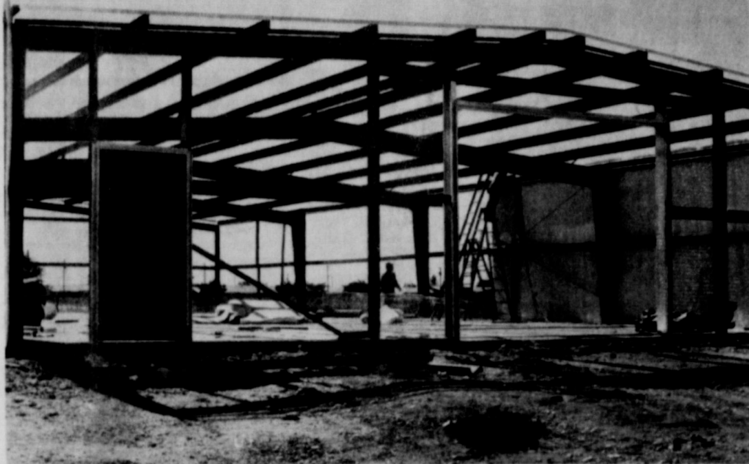
SHOW BARN GOING UP---A new community service building--planned for use as an ag show barn and various other functions--is taking shape on 20th street, near Babe Ruth Park. Officials are hoping to have the building ready for the Slaton Pig Sale, scheduled at 6 p.m. Tuesday, Oct. 26. The ag committee of Slaton Chamber of Commerce spearheaded the project to secure the community service building.
