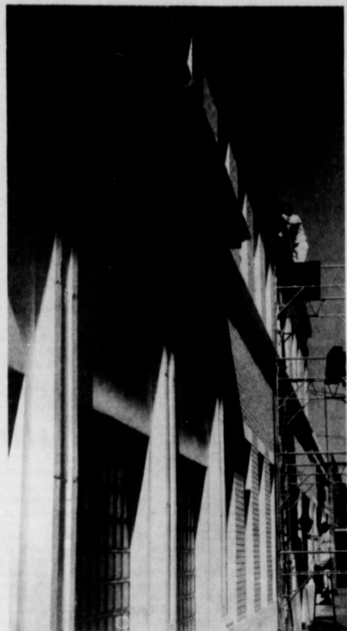
BRIGHTER THAN WHITE --A number of improvements have been accomplished on Slaton business firms the past few months, and one of the latest is a new white paint job on the Slaton Savings & Loan building. The photographer caught one of the painters high atop a scaffold in this picture.
