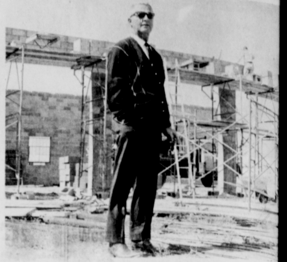
NEW COUNTY SHOP---The term "barn" will be outdated when the new Lubbock Maintenance Shop is completed here in Slaton. County Commissioner Max Arrants is looking over the shop as construction moved well along this week. Shop is on old US-84 and Cemetery Road, on land purchased from the City of Slaton. (SLATONITE)
