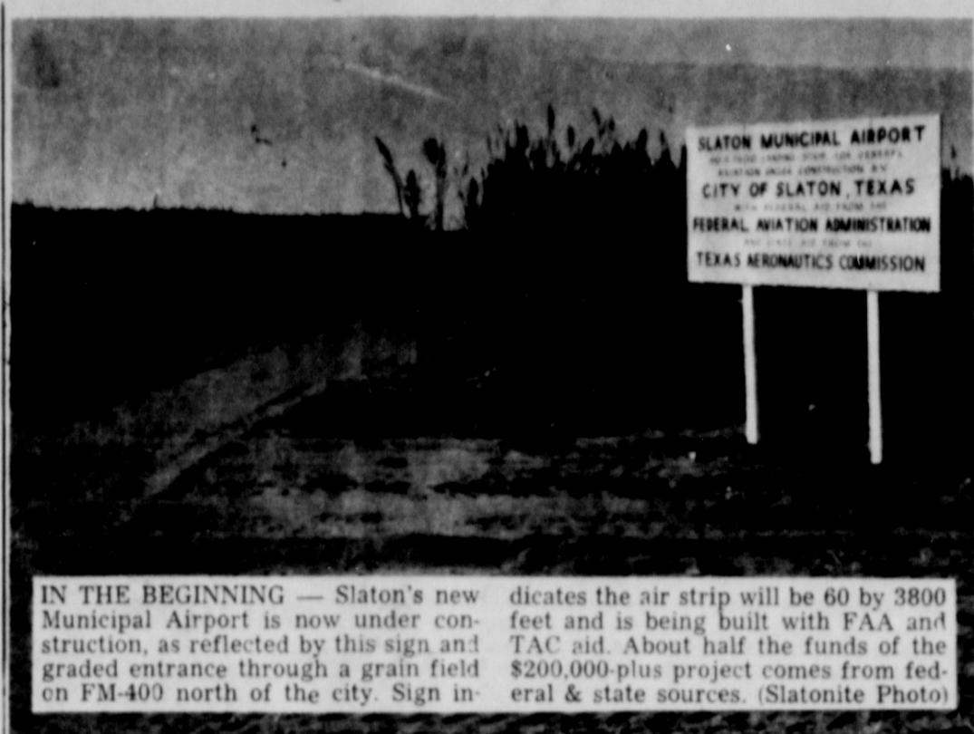
IN THE BEGINNING — Slaton's new Municipal Airport is now under construction, as reflected by this sign and graded entrance through a grain field on FM-400 north of the city. Sign indicates the air strip will be 60 by 3800 feet and is being built with FAA and TAC aid. About half the funds of the $200,000-plus project comes from federal & state sources. (Slatonite Photo)
