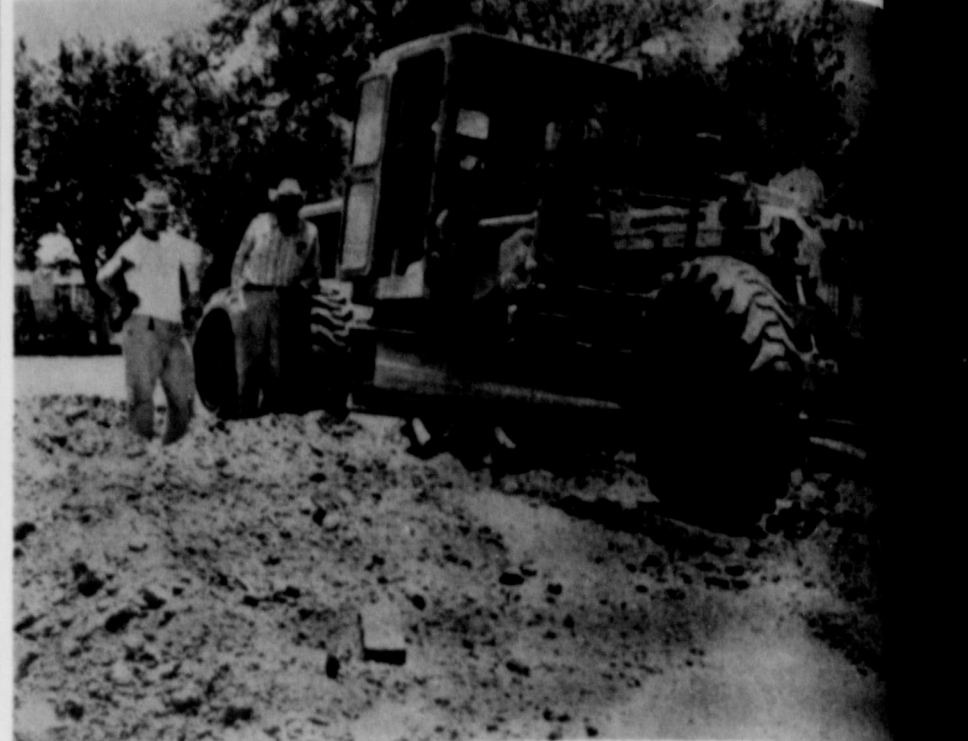
PAVING PROJECT UNDERWAY — Slaton's 1965 paving project, which will include about 80 city blocks, is now underway. This scene at 13th St. and Garza was taken Tuesday by employees of Pioneer Pavers working readying the street for paving. (SLATONITE FILE)
