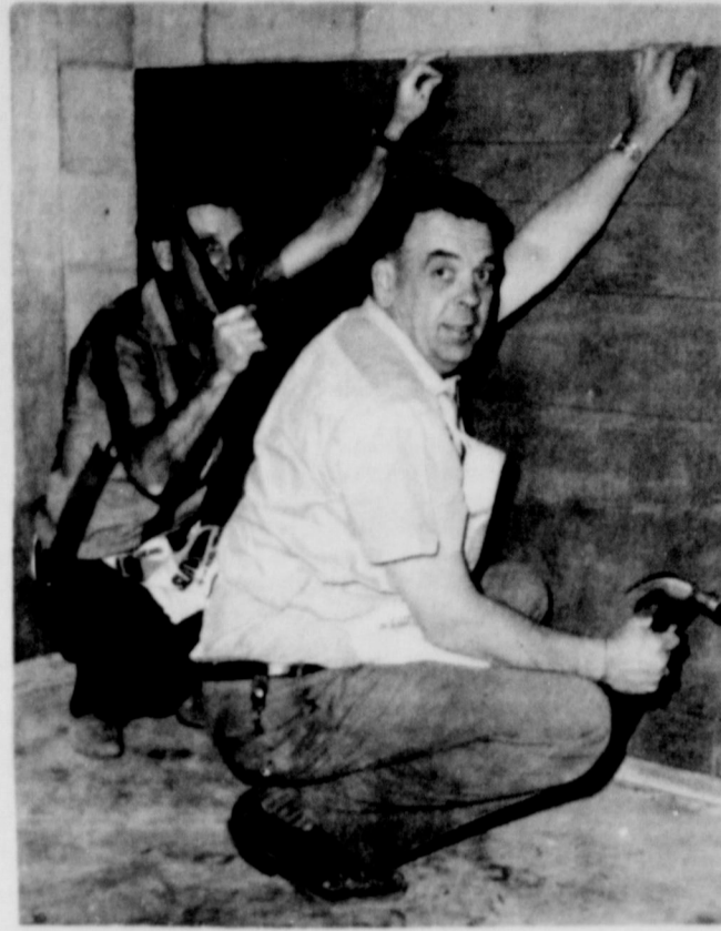
INSTALLING PANELING??--Two volunteer workers are shown installing paneling in Slaton's new youth center building. Ray Ayers, left, may not hit the nail every time and a few seconds later, Bud England, agreed. From the looks of the building, they are pretty good with hammer and nails. (SLATONITE PHOTO)
