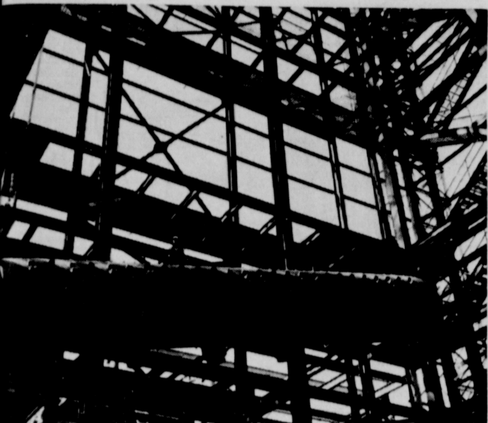
THE GROW--Continued construction on a 210,000 kilowatt generator at Nichols Station, northeast of Amarillo, is part of Southwestern Public Service Company's $20 million improvement program for 1967. Pictured is the installation of a 225,000 lb boiler drum for the new generating unit.
