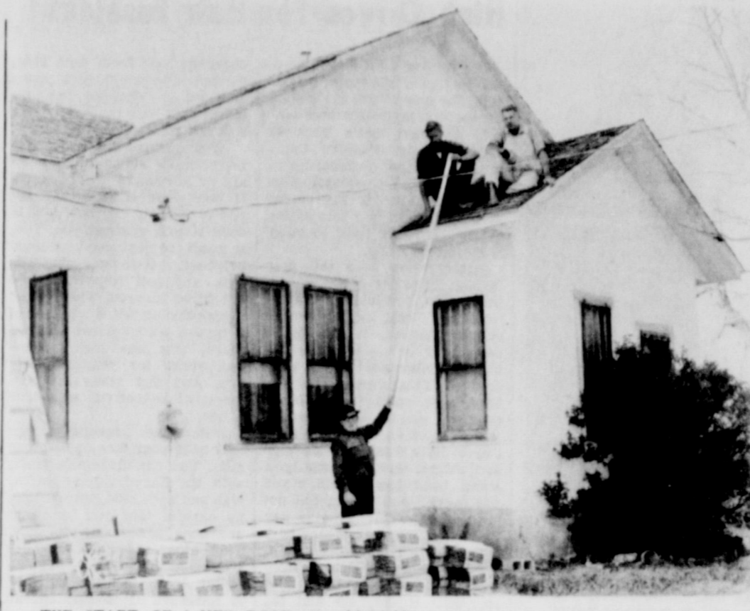
THE START OF A NEW ROOF--Harold Fishback and his father, Loyd Fishback, carpenters for Dickie Construction and Slaton Lumber Co., are shown on the roof of the home of Miss Ethyl Spooner. Ray Dickie is shown standing beside the new roofing to be put on the house. The men are donating their time so Miss Spooner may have a roof that doesn't leak. Other men are needed to help complete the job. See story in today's Slatonite. (SLATONITE PHOTO)
