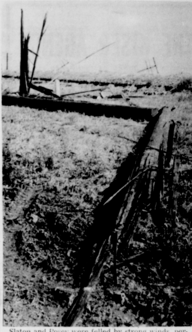
Slaton and Posey were felled by strong winds, perhaps a small twister. Tuesday night. Shown is one of the 11 poles knocked over, some falling across Santa Fe tracks.
