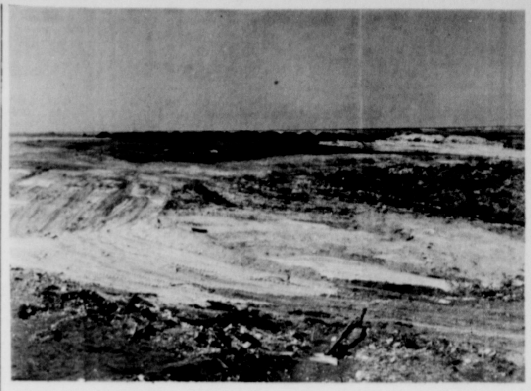
STILL IN THE ROUGH --Slaton's new municipal golf course is still "in the rough" but the links layout is beginning to take shape. This photo, made from the approximate position of a tee box, shows ground work being done and a rough "green" in the left background. The canyon will provide a scenic view on the 9-hole course. (SLATONITE PHOTO)
