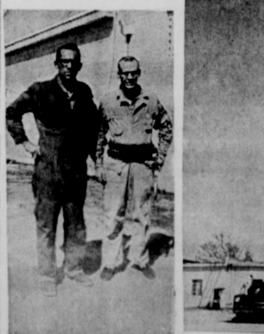
Pictures here show repairs being made to the radio antenna at Slaton Police Headquarters. A connection had been broken by vibration in recent high winds. Lubbock Fire Department sent their ladder truck with 85-foot extension ladder and the Department sent Radio technician Bill Williams and dispatcher Gary Hagermiller to do the work. Pictures show Williams at left, Hagermiller at right. The other was taken as Hagenmiller was being pulled up to the top of the mast. Police Chief Joe Martin was unwilling to allow anyone to try to climb the aluminum mast.
