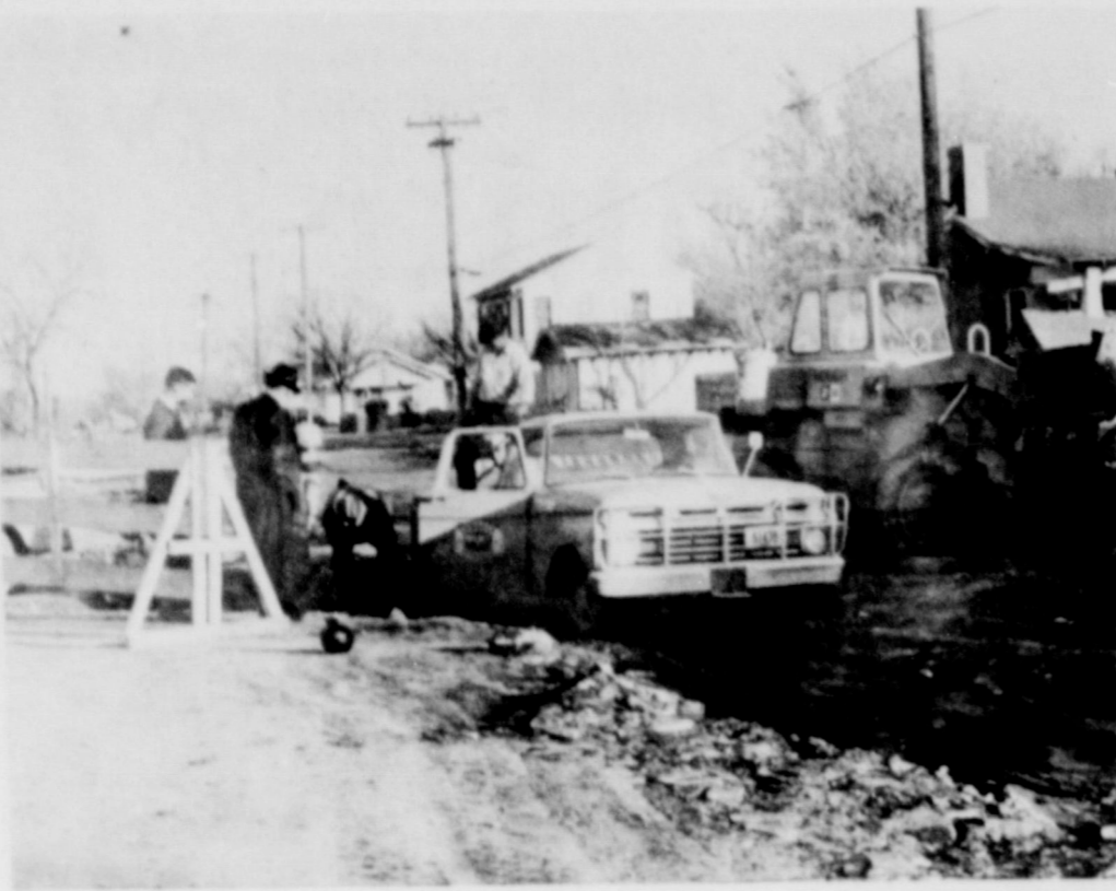
WORKING ON DIVISION--The construction work on Slaton's Division Street was proceeding this week, and the contractor was expected to "shoot" the primary hot asphalt mix to the street in the next few days. Mayor Jonas Cain and City Secretary Bobby Sokoll are pictured at left as they look over the work. (SLATONITE PHOTO)
