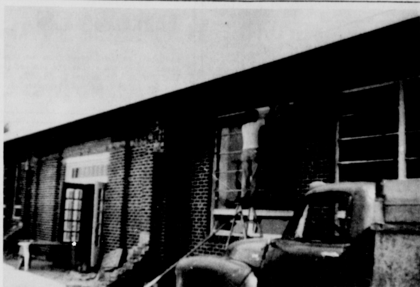
NOW ONE STORY--Pictured above is the renovated Junior High Building, now a one-story structure. The old building was three stories. Shown installing the windows is Phil Corona, an employee of the School District. The new school should be ready for the new term opening.
