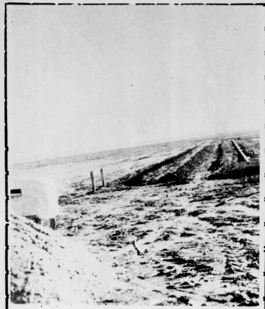
MOTEL UNDER WAY - It may take a bit of imagination to see the faint outline, but this is the beginning of a motel-shopping center being built just west of Muleshoe by Mr. and Mrs. Bill Shankles. This is the first phase of a $3. million program. This contract calls for an 18 unit motel, office spaces for rent, a coin laundry and a permanent mobile home park. M. E. Lee & Son has the contract. (Journal Photo)
