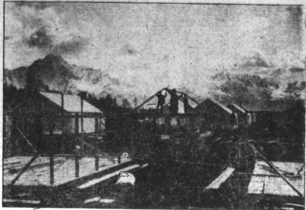
In the shadow of snow-capped mountains 500 CCC workers are building the tent city for midwest farm families the federal government is transplanting in the fertile Matanuska valley of Alaska. This is the first picture of the pioneer town where 67 Minnesota families already are settling. (Associated Press Photo)
