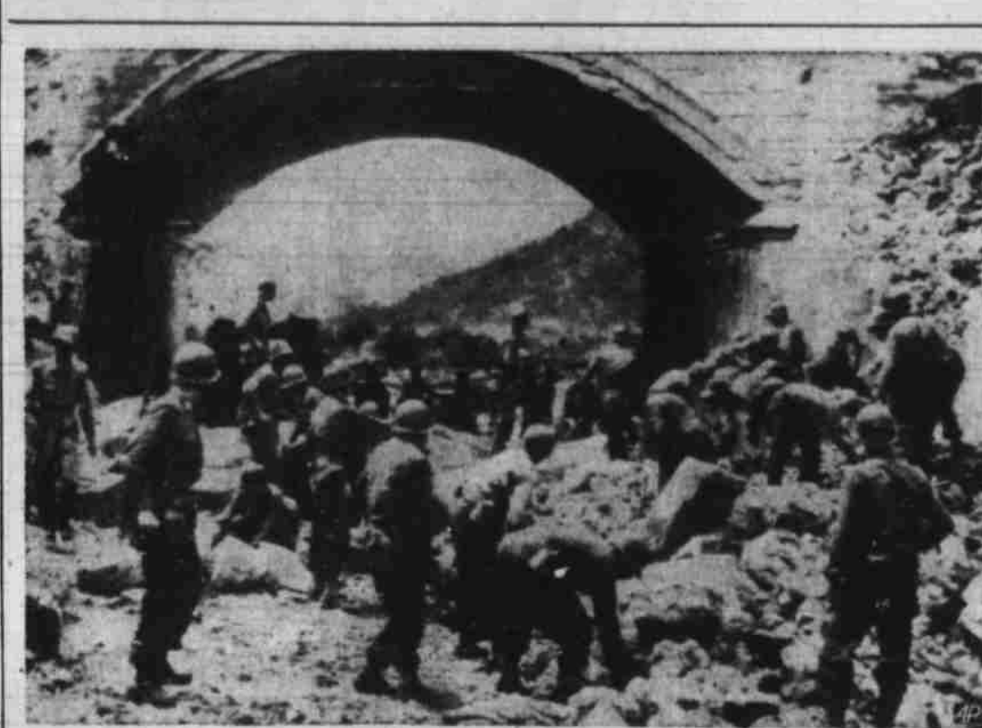
Engineers Clear Way—American engineers clear the rubble from the Applan Way under a railroad bridge near Itri, Italy, as the new Allied offensive continues to drive the Germans backward. (AP Wirephoto from Signal Corps Radio.)
