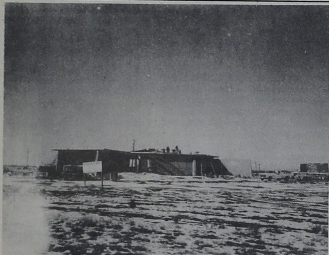
Work continues on the new American Bank of Commerce at Wolfforth building just on the outskirts of town.
