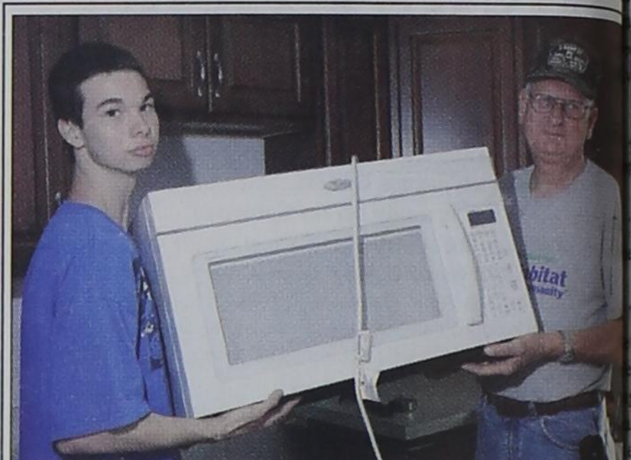
Rockwall High student Jake O'Neill, 16, and Rockwall resident Jim Otto, a three-year volunteer with Habitat for Humanity, prepare to install a microwave oven at the local Habitat build site on Peter's Colony. Rockwall Area Habitat for Humanity also recently broke ground on its next house also on Peter's Colony. To volunteer or for more information about Rockwall Habitat, visit rockwallhabitat.org . Photo by Roy Heath/Rockwall County News
