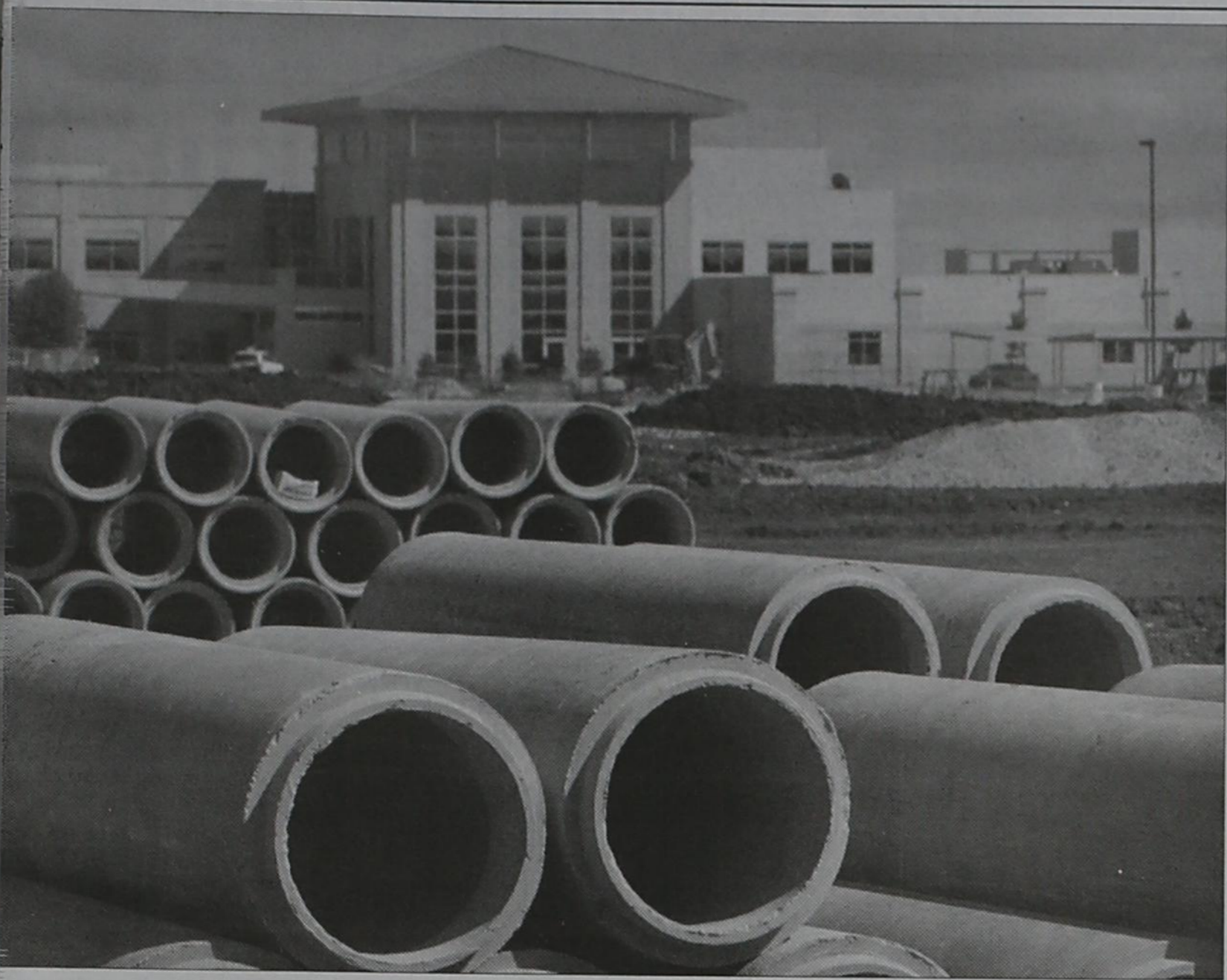
Work on the expansion at Presbyterian Hospital of Rockwall. (Staff Photo by Tim Burnett)
