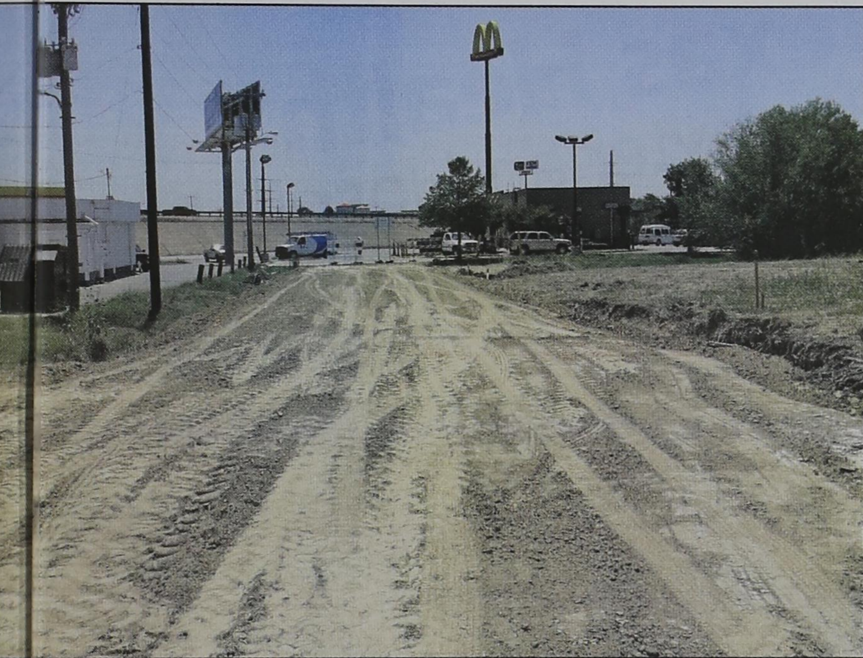
Work on the new exit road for the Royse City McDonald's is well advanced. When the Erby Campbell overpass construction begins, one of the first things the Texas Department of Transportation engineers proposed was to make both the north and south service roads one-way to all traffic. The north service road will be westbound from the Shell Station at Elm Street (FM 35), while the south service road will serve eastbound from Circle Lane. Typical TxDOT procedures are to work on the road adjustments first, including the relocation of utility lines prior to the start-up of construction. Once service road adjustments have been completed, customers arriving at McDonald's via the new road westbound will be directed to depart behind the Shell station and exit onto South Elm Street.
