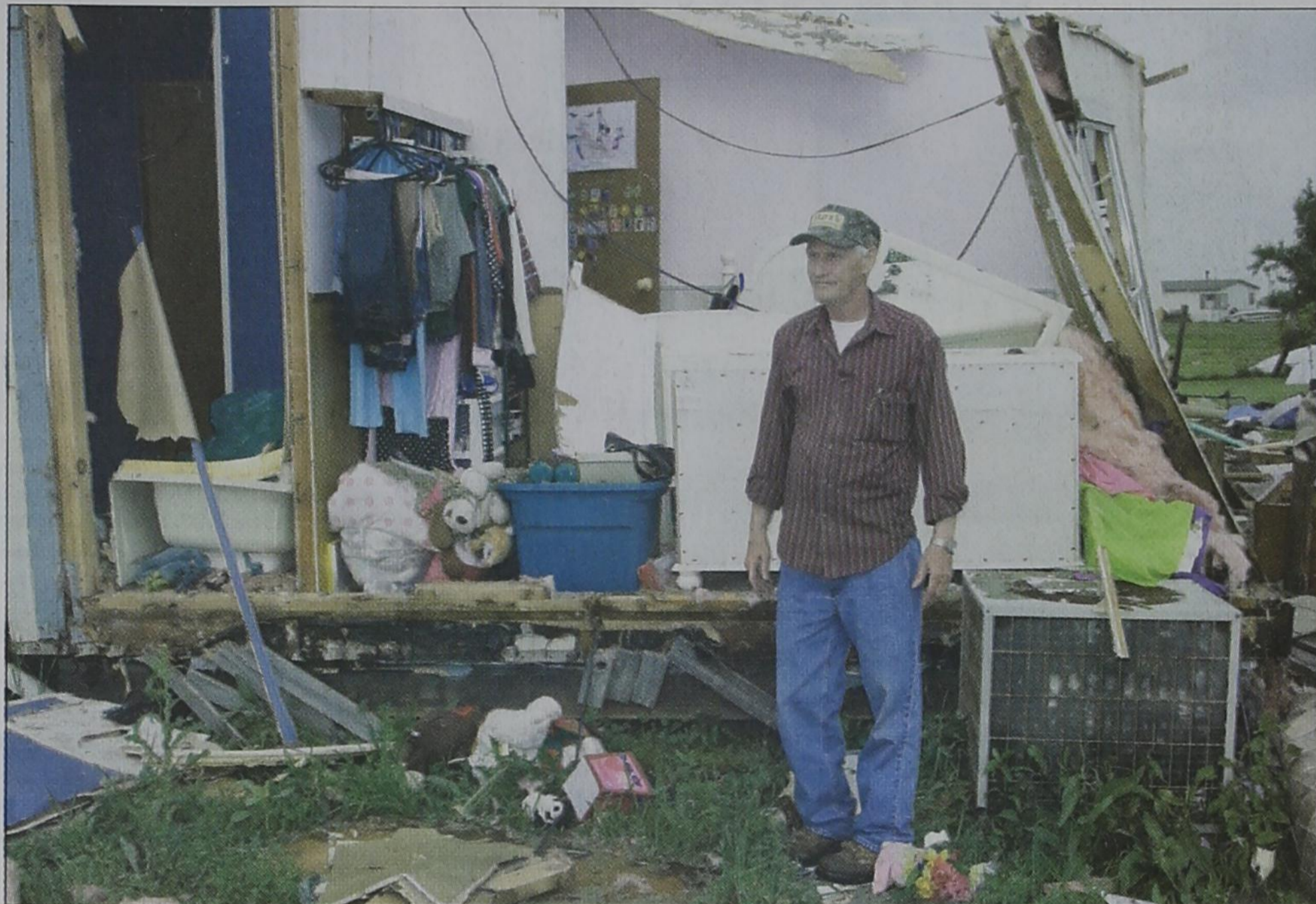
Royse City resident Billy Miller inspects the damage to his home on Honey Creek Drive after last week's tornado. Miller and his family have lived in the home for more than 20 years. Photo by Tim Burnett/Rockwall County News
