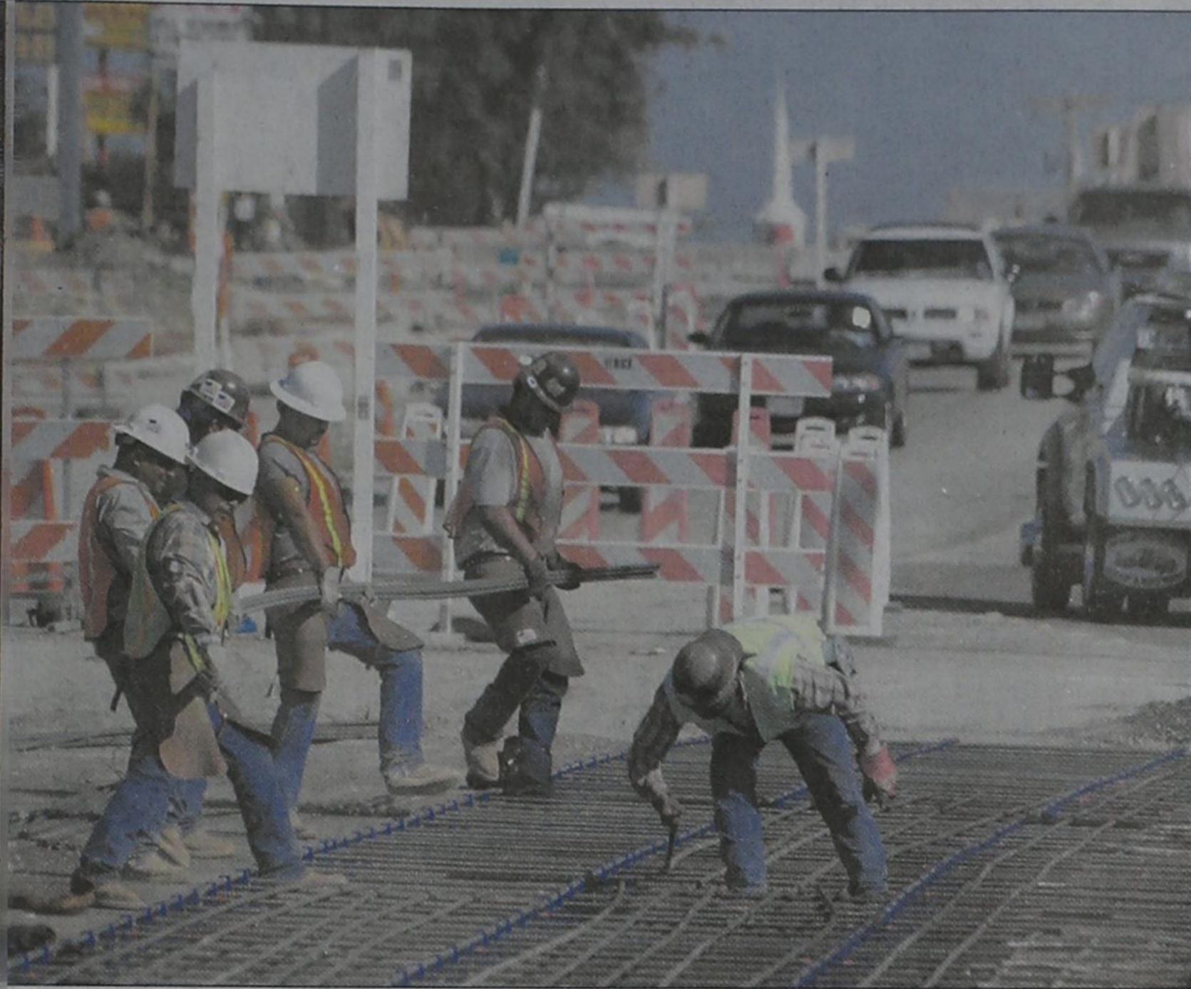
Construction crew members prepare to pour cement last Tuesday at the north side intersection of Goliad and I-30. Photo by Tim Burnett
