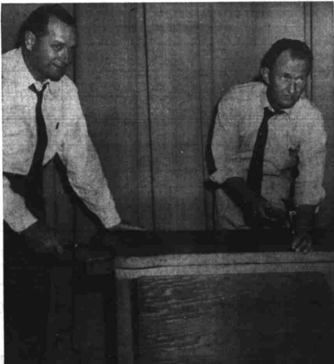
SET BUILDERS — Practicing some of their do-it-yourself skill, Luin King, left, and J. T. Wilkinson work to help on the sets for the minstrel show. This is an annual event of the Lions Club, with proceeds going to their Charity Fund, and most of the members take part in some way.
