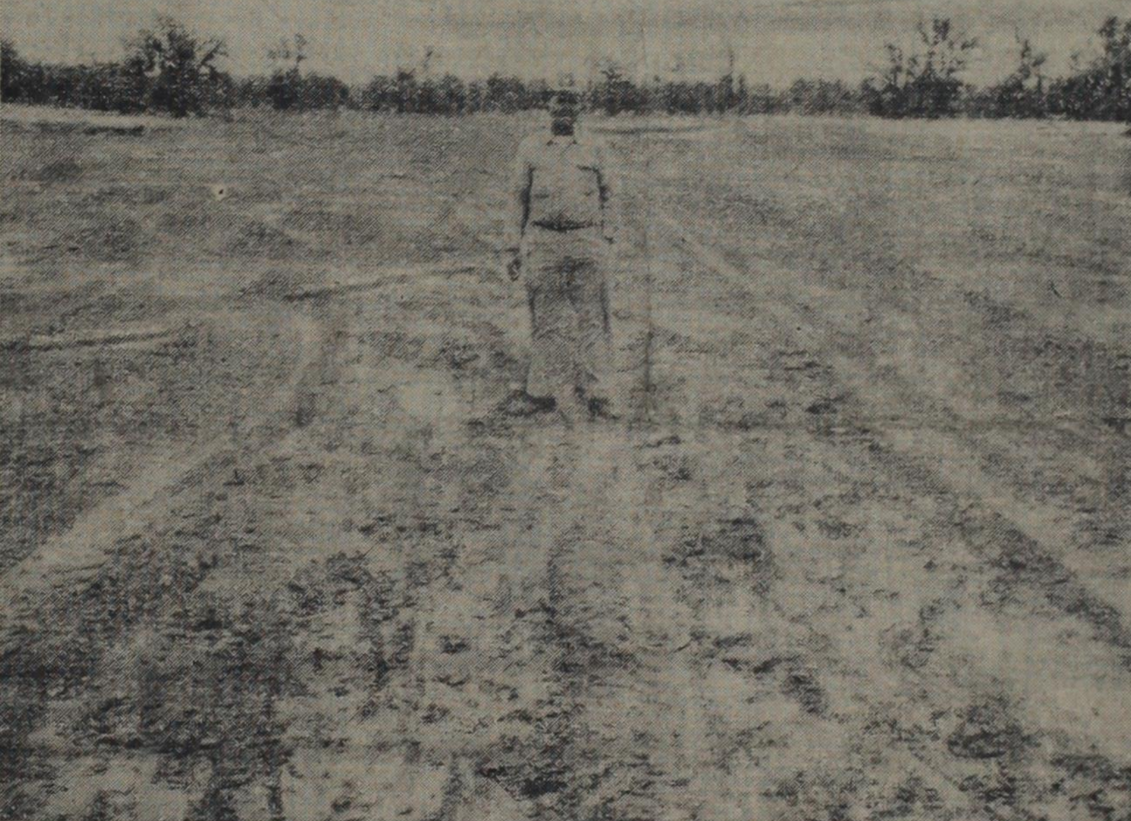
shaped and ready for sodding to coastal bermuda grass. John Lee, Jr., Rising Star conservationist, is shown in the top and below, Olin Lee, May, Texas, contractor.
