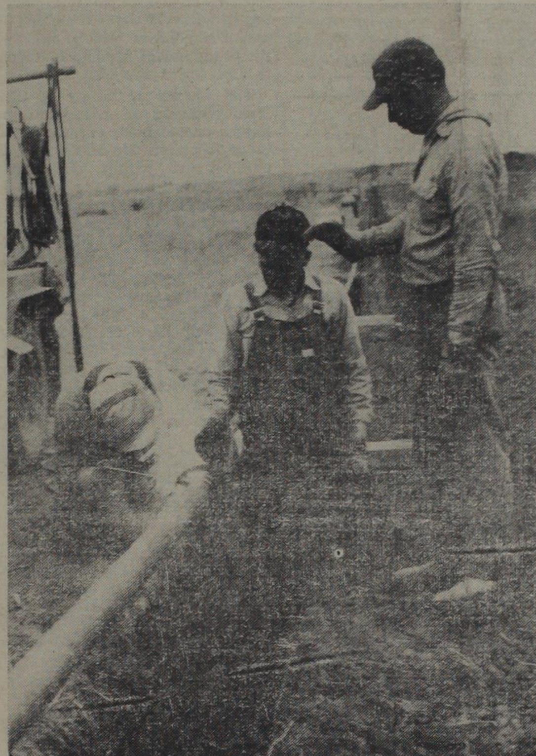
Through this 3-inch pipeline which welders of the Henson Construction Company, Cisco, are shown putting together, gas from the Moore 5,000,000-foot gas well near May will shortly be flowing to the stoves and ranges of Rising Star. Work was resumed Wednesday after a lay-off because of ice and bitter cold.
