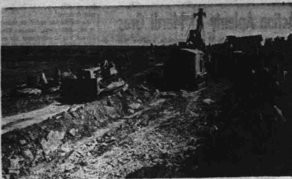
COLORADO WATER PROJECT UNDERWAY—Earth-moving machinery is kept rolling 22 hours a day on the new Morgan Creek reservoir four and a half miles southwest of Colorado City. The dam will back up a lake seven miles long, will make possible a steam-electric generating plant for the Texas Electric Service company, and will provide Colorado City with badly needed water supplies. (Photo by Jack M. Haynes).
