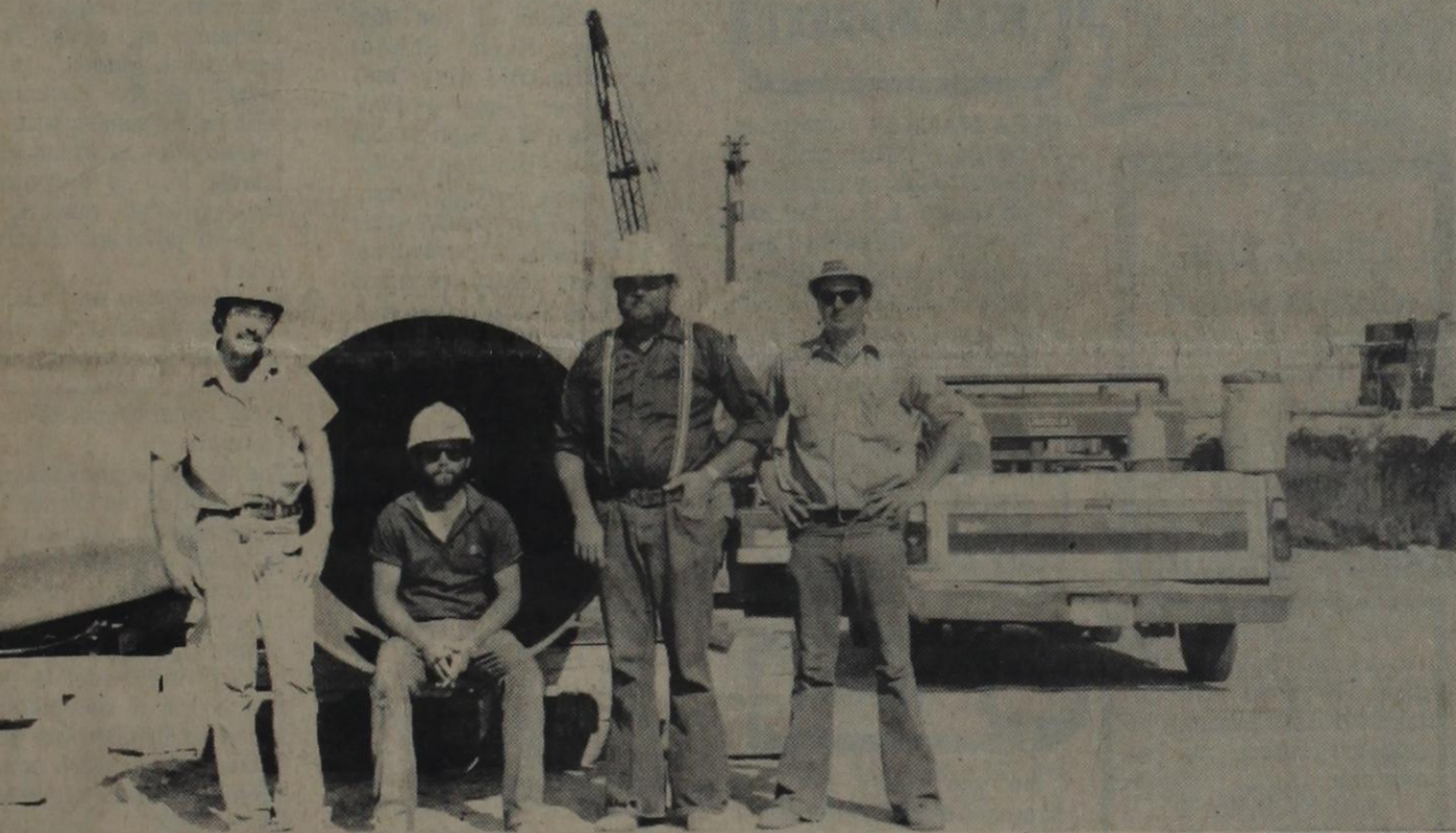
These men are busy working on the underground storage facility for Odessa Natural. They are left to right: Randy Flowers-Construction Super-
