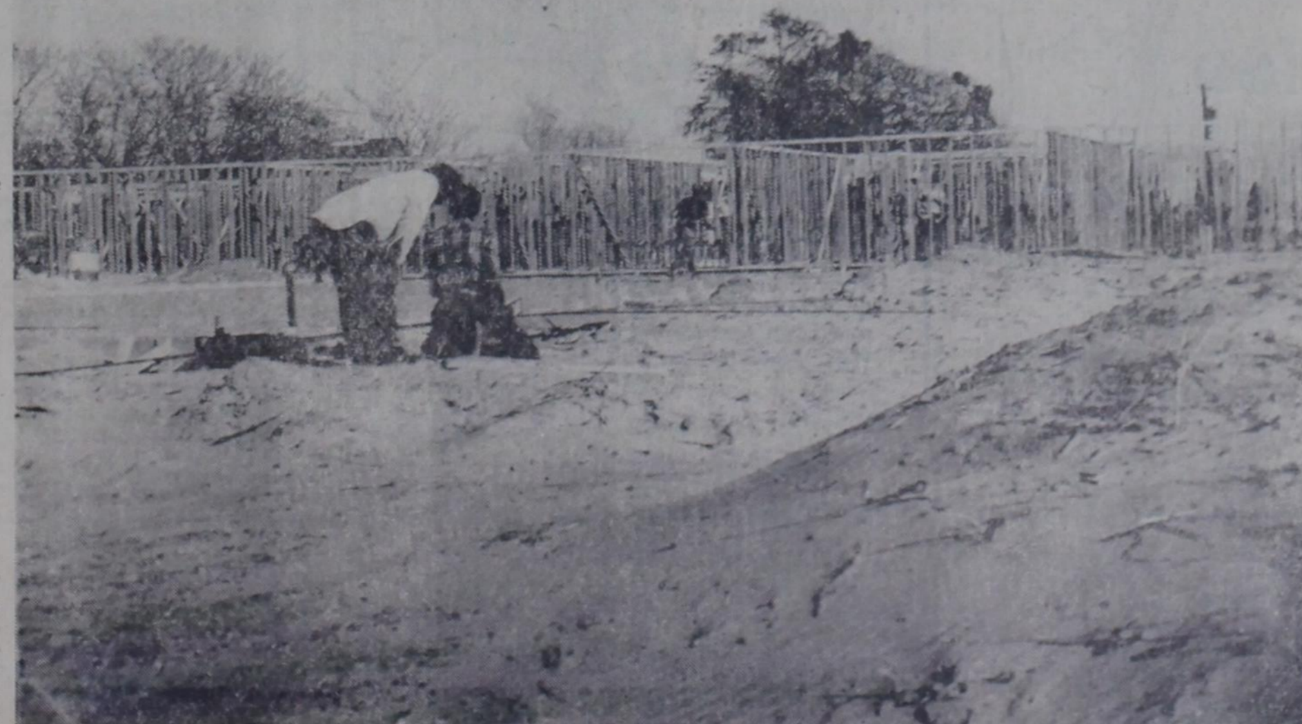
GOING UP—Framework for the new First Baptist Church is rising rapidly from foundations laid on the site of the church which was destroyed by fire last October. This view shows studding for the edu-
