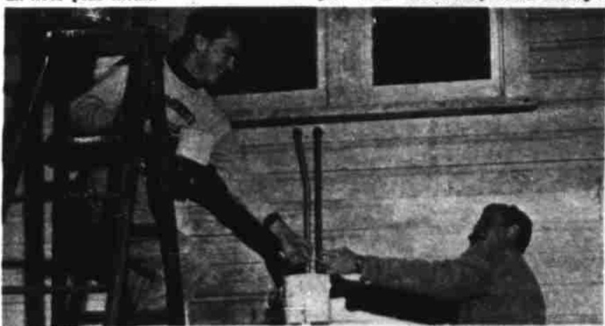
Job opportunities on college campuses are varied, but it is up to the student to find out about them. Here a couple of University of California freshmen turn their talents to painting school buildings.
