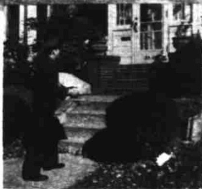
Faulty steps invite a fall and possibly a costly damage suit.
