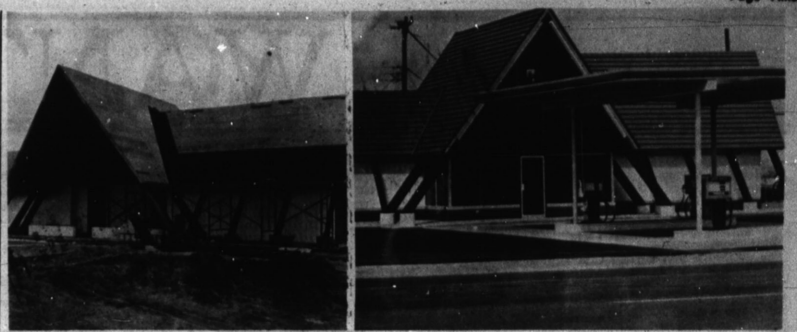
NOW AND THEN — Work on a service station on 25 Mile Avenue is progressing rapidly and soon will look like the finished product pictured at right. Station owners said the Hereford business will be a replica of this one in Amarillo. (Hereford Brand Photo)
