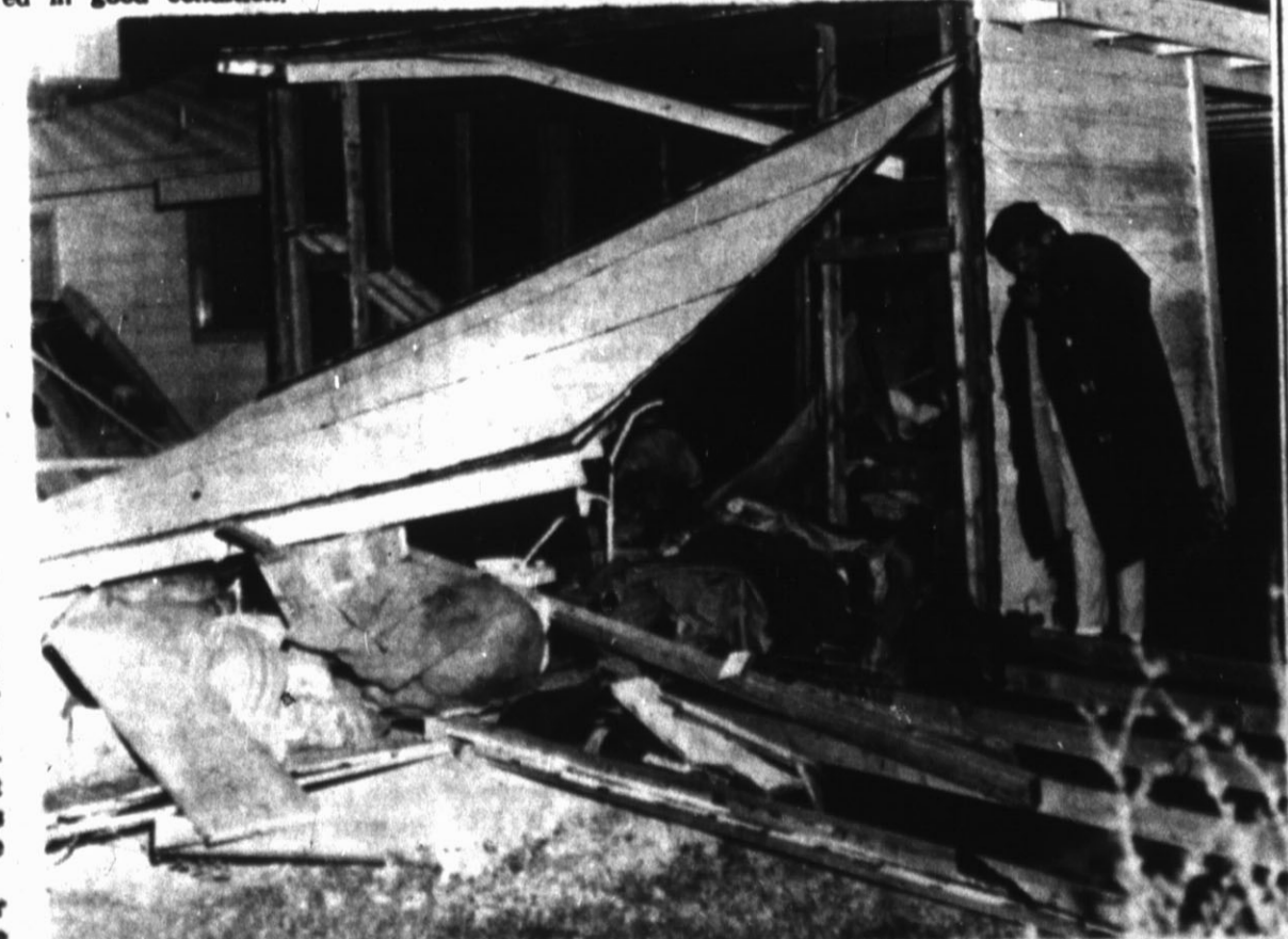
RESULT OF BLAST—Hereford Marshall Terry Hoie examines damage caused by an explosion here Sunday night which sent three persons to Deaf Smith County Hospital. The blast, apparently caused by a small butane stove, flattened this storage shed at the rear of a corport of the E. H. Prieto residence, 439 Ave. G. (Staff Photo)
