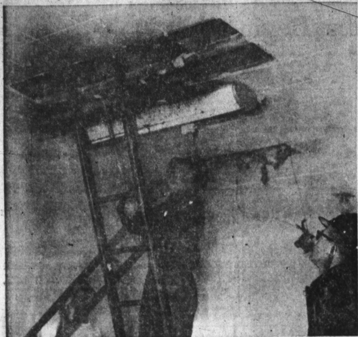
FIRE'S ORIGIN is probed in the ceiling of the building's east wing, the I. O. O. F. Hall Sunday about 1 p.m. causing damage estimated at $2,000. The electrical short circuit caused a fire (Staff Photo)
