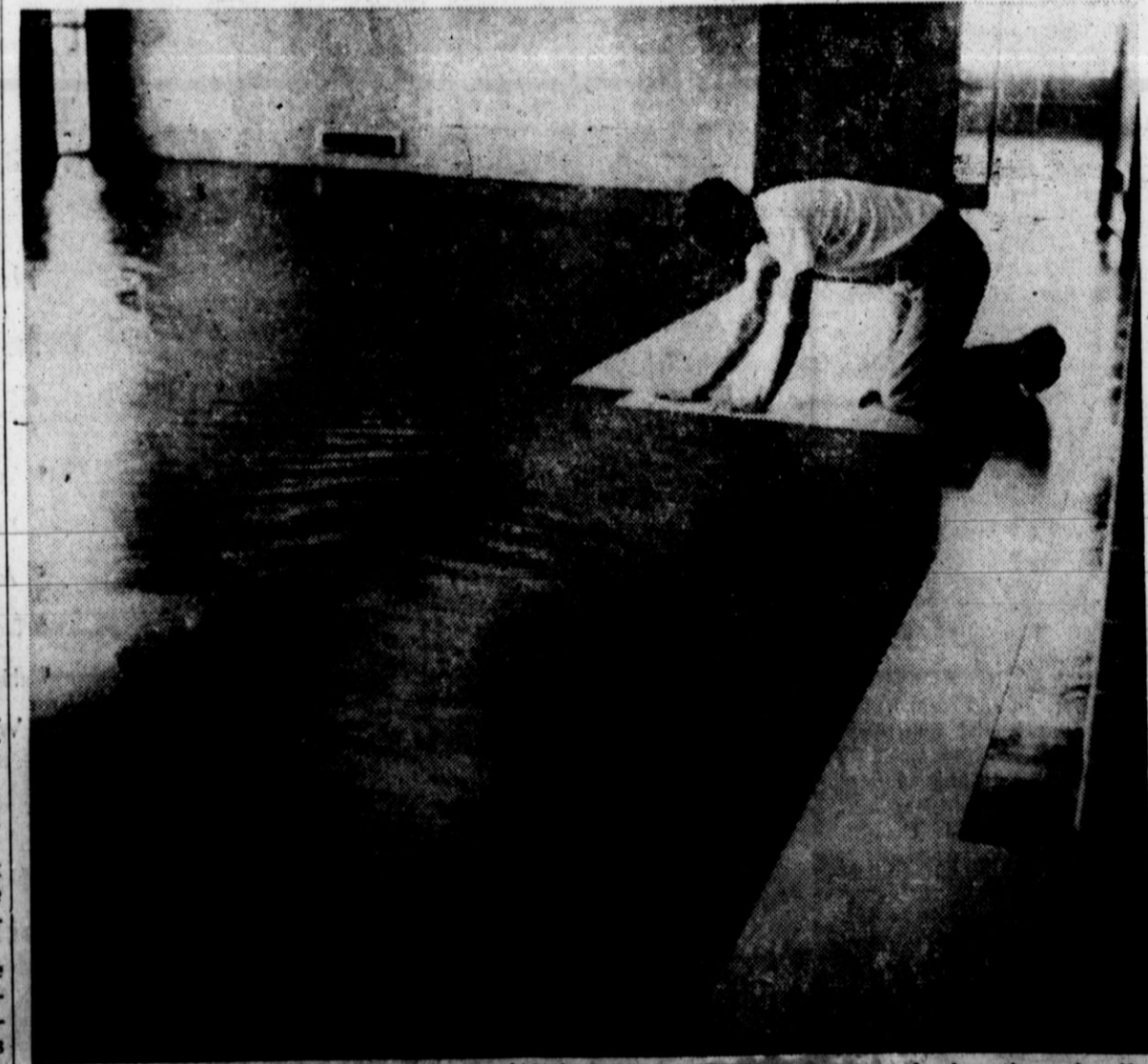
TILE SETTERS had a long way to go Wednesday at the new Northwest School. The flooring and some of the finishing work was all that was needed on the finished building. School officials transferring the school's temporary classrooms at Central Church of
