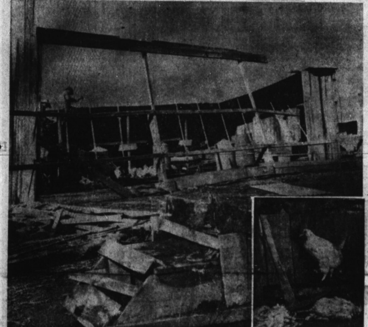
STORM DAMAGE—Heavy winds ripped the roof off Ken Rudd's chicken house on his farm nine miles west of Hereford Friday afternoon...
