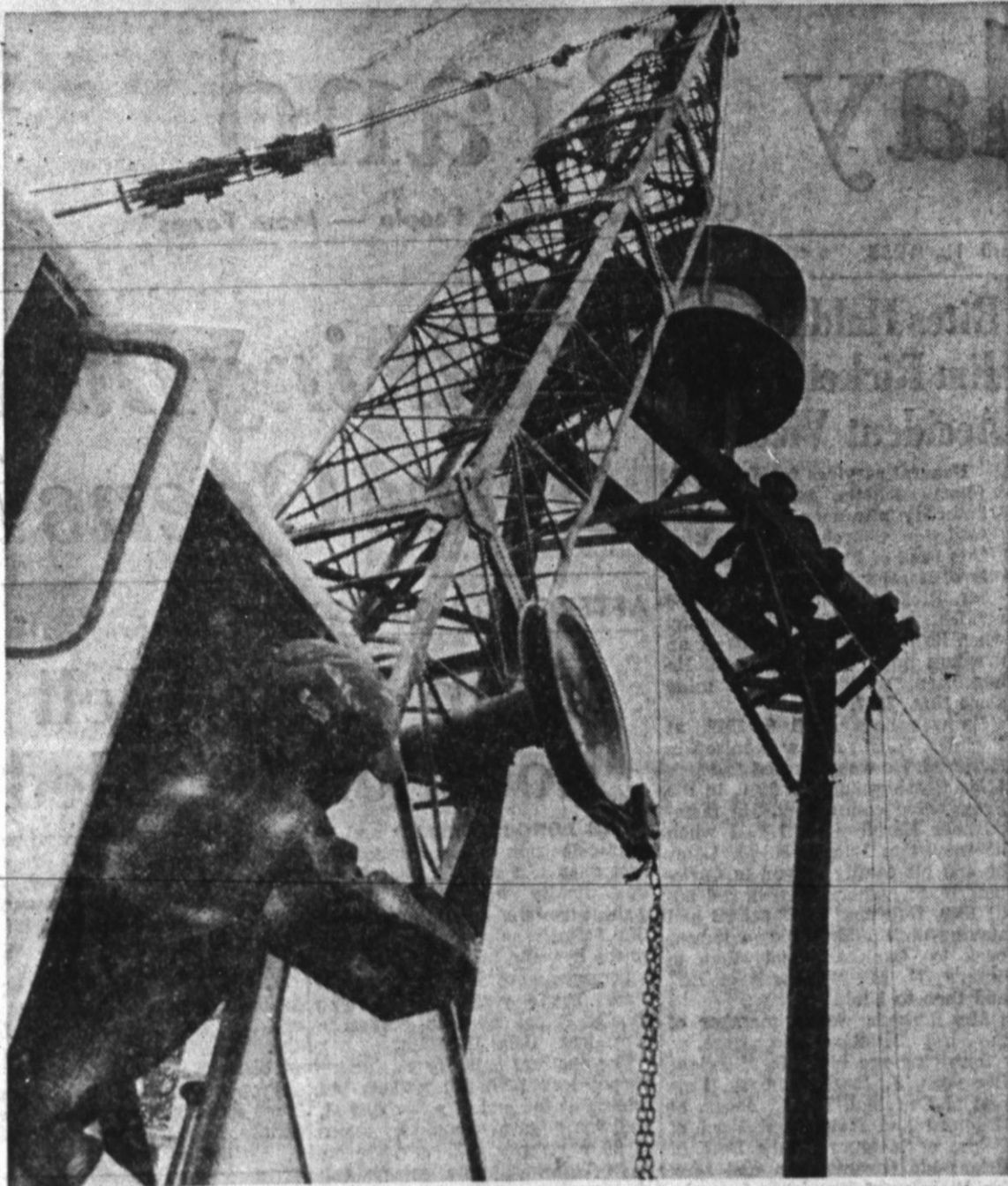
INSTALLING TORNADO SIREN—Two tornado warning sirens were installed by the city this week, one atop the city hall and the other in the alley between H and I Avenues south of Union. Though no date has yet been set for testing of the units because of a delay in wiring due to wet conditions, the signals which will be used are: alert (first warning) solid blast lasting three to five minutes; next signal (take over) will be an undulating sound, up and down, for three minutes. No all-clear signal has been designated. The alert will be sounded when tornadoes are actually in the area. "There'll be no trouble telling when the tornado warning siren goes off," stated city manager Dudley Bayne, "they're a lot different from the fire siren and a lot louder." (Staff Photo)
