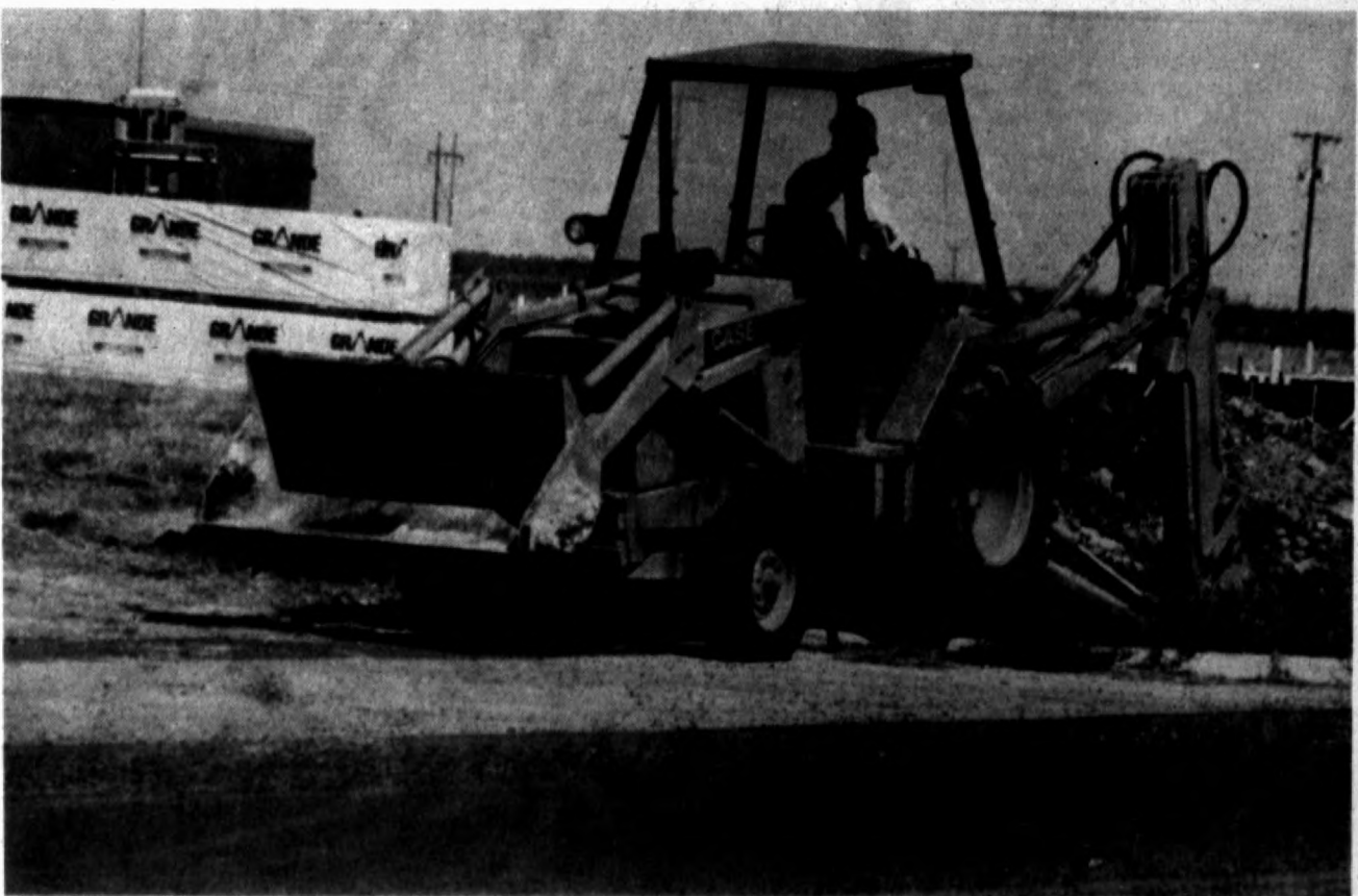
Installing water line at nursing home site City employees work on a new water line for fire hydrants in front of a new nursing home in northwest Hereford. Work is continuing on the site, with concrete work to begin soon.
