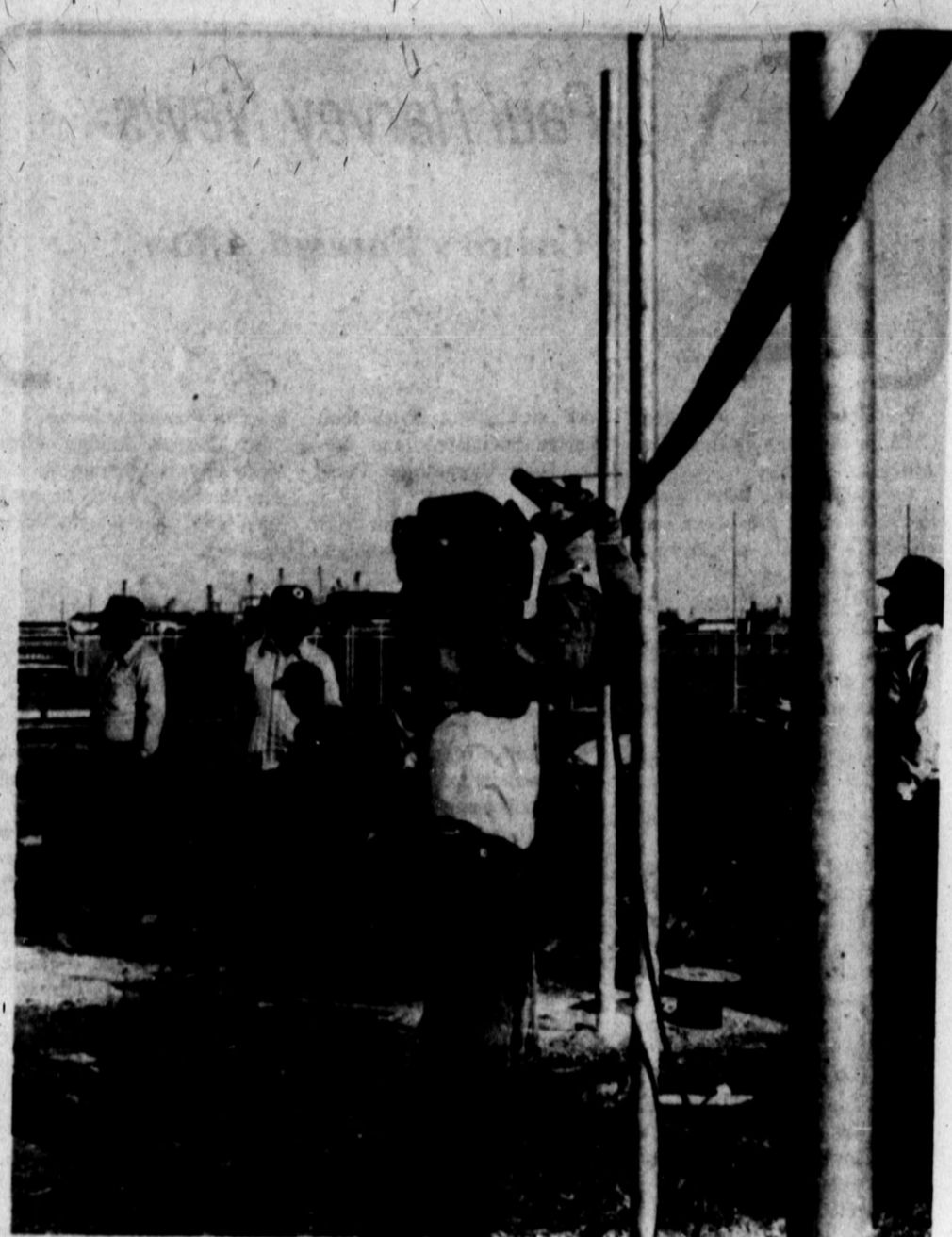
Progress Volunteer workers construct fence at the Kids Inc. baseball complex Tuesday. Pioneer Natural Gas Co. of Hereford is donating welding equipment and manpower for getting the fences up at the complex. A workday will be held at the complex Saturday, and Chuck Cosper of Kids, Inc. encourages everyone to bring rakes, shovels and hoes for the work session. Although the complex is going up at a rapid pace, Cosper pointed out that much remains to be done in order for youngsters to open the season on the new ballfields May 8. [Brand photo by Jim Steiert]
