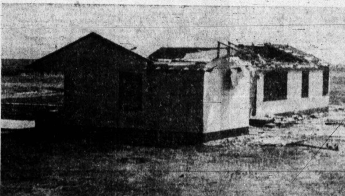
THIS VIEW OF the W. S. Dameron home shows the overall picture of how Monday evening's twister tore the roof off the place, causing damage estimated from $3500 to $4000. This view was taken from the southwest corner of the yard. Brand Staff Photo.
