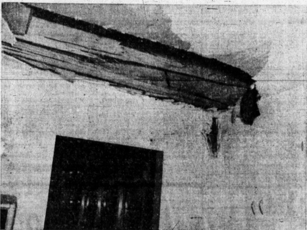
THE CEILING of the kitchen of the ranch home of Mr. and Mrs. W. S. Dameron was damaged as shown in the above photo. Ceiling damage to the adjoining living room was limited to a hole where a piece of 2x4 was driven through it.—Brand Staff Photo.
