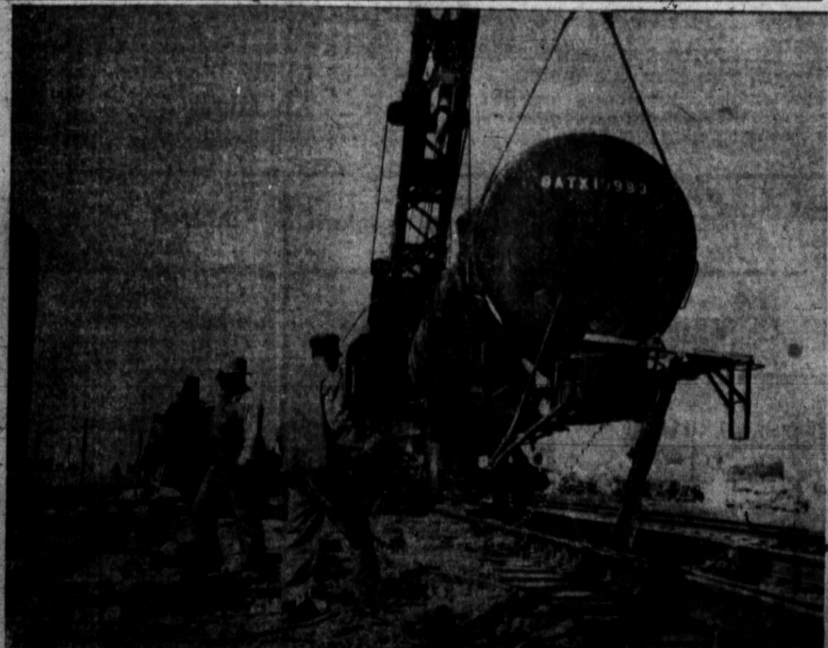
SALVAGE OPERATIONS for the Santa Fe freight car derailment early Sunday morning are shown in the above picture. Here the derailed gasoline tank car is being lifted onto the tracks as workmen in the rear of the photo are pushing a set of trucks under the end of the car in the right corner of the picture. Brand Staff Photo.
