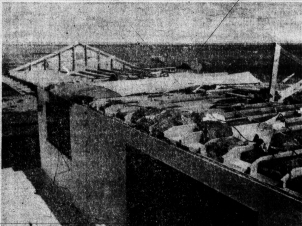
A CLOSE-UP of the tornado damage to the ranch home of Mr. and Mrs. W. S. Dameron Monday shows how the twister cleaned off the roof, leaving the majority of the insulation bats still in place between the rafters. Brand Staff Photo.
