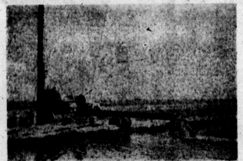
Pomona Pump installed last April for E. G. Wright.
