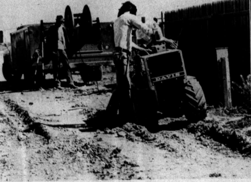
CABLEVISION WORK CONTINUES —Burial of underground cable for cable television service in Northwest Hereford nears completion along with installation of aerial cable in other parts of the city. The system is expected to be in service for the northeast portion of the city around June 1, with the northwest part of the city ready for service shortly afterward.
