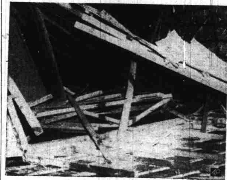
STORM DAMAGE AT MABANK, TEXAS—This is one of several buildings wrecked by a windstorm which struck Mabank, in East Texas. Mabank was one of several northeast Texas communities struck by windstorms the night of April 29. (AP Photo.)
