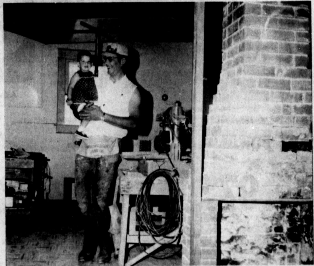
A REST IN RENOVATION is taken by Devers to play with his small daughter in the kitchen, where he applied wallboard to the ceiling. Some of the tools which make his work easier are on the bench where he leans. Repairs are scheduled for the fireplace which faces into the family room area.
