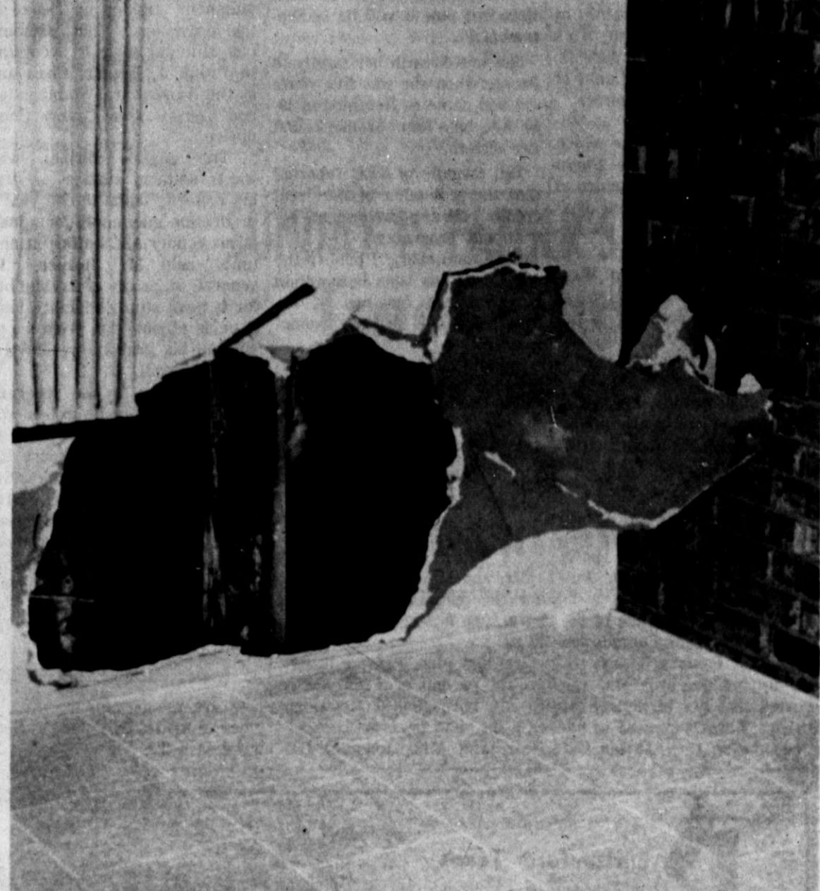
FREAK STREAK — This gaping hole in the interior of the Camp Fire Lodge was believed to have been the result of a freak bolt of lightning sometime Monday night or early Tuesday morning. Damage was confined to the attic and interior of the building. —Staff Photo
