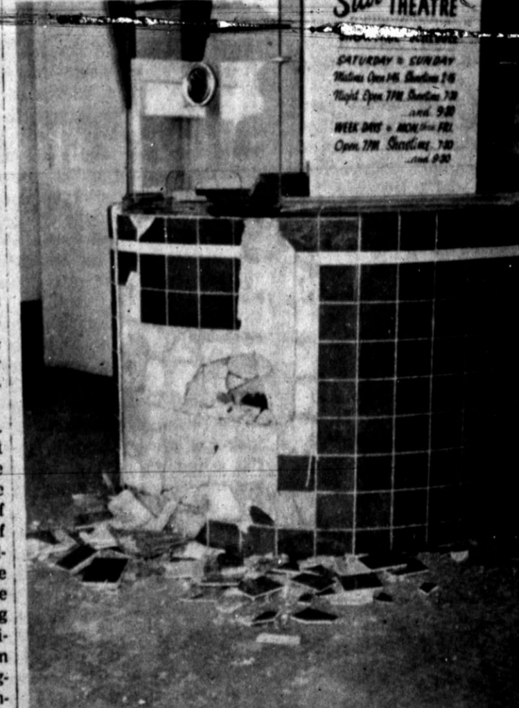
BRAKE FAILURE — An estimated $550 damage was reported to the box office of the Star Theatre Monday night. A car driven by Bill Amaro, 606 W. 2nd St. attempted to park in front of the theatre when his brakes failed, causing the accident. Amaro then backed the car to W. 3rd St., jumped the curb and struck the Ben Franklin Store, a block away. —Staff Photo
