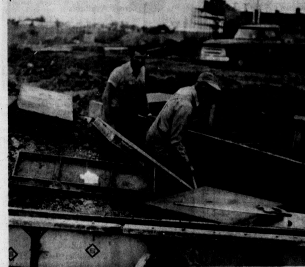
TIERRA BLANCA RISES — No, not the Tierra Blanca Creek, but the Tierra Blanca Elementary School which is being constructed on South Lane, near Country Club Drive. Des-
