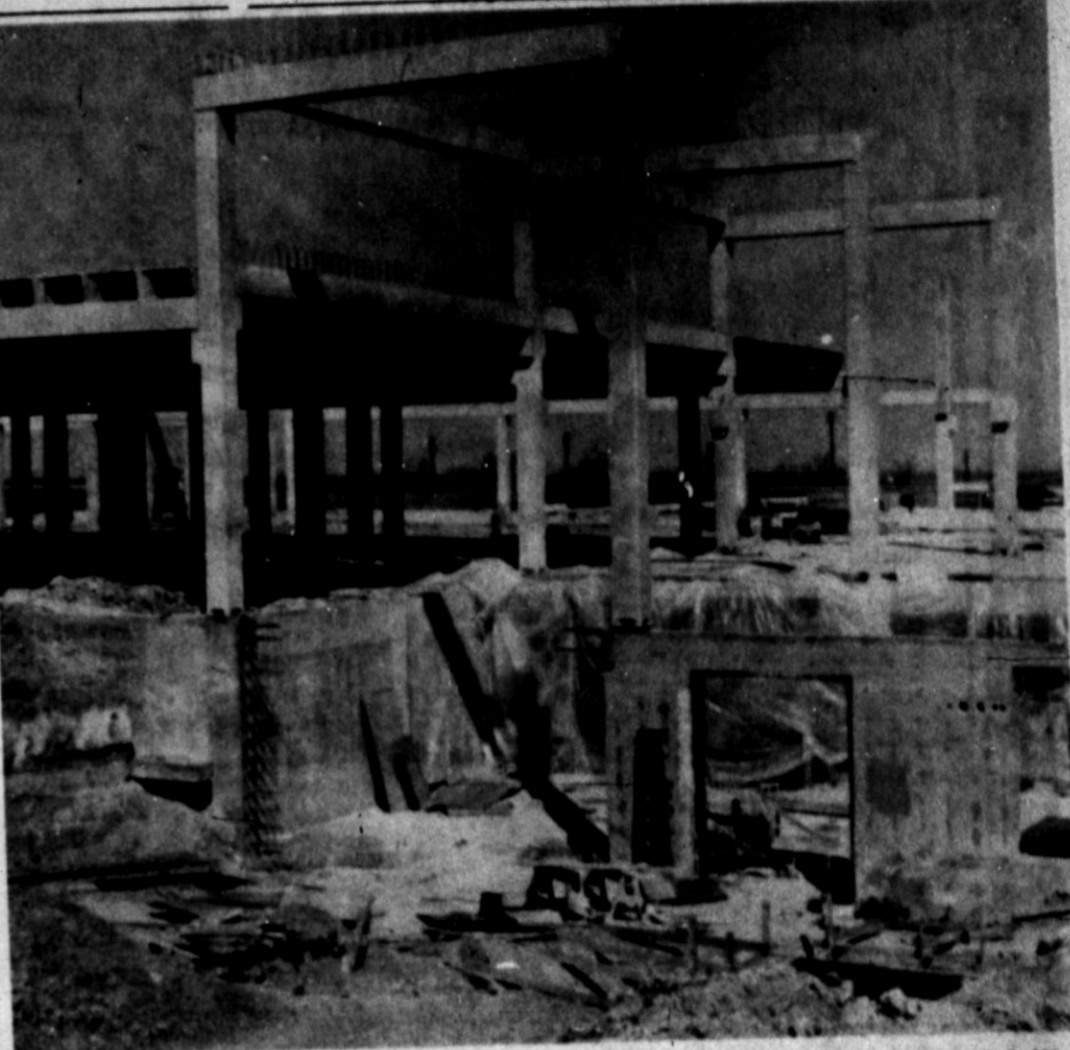
STRUCTURES UP — Concrete framework at the Wilson and Company meat packing plant's main building has been erected recently, while touch-up work is being completed on the basement
