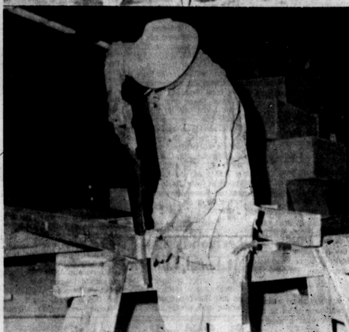
INSIDE THE WILSON PLANT — Shown above are only a few of the many workmen striving to meet the January 1, 1970 deadline of completion of the Wilson Packing Plant. The plant is located two miles west of Hereford on U.S. 60. —Staff Photo
