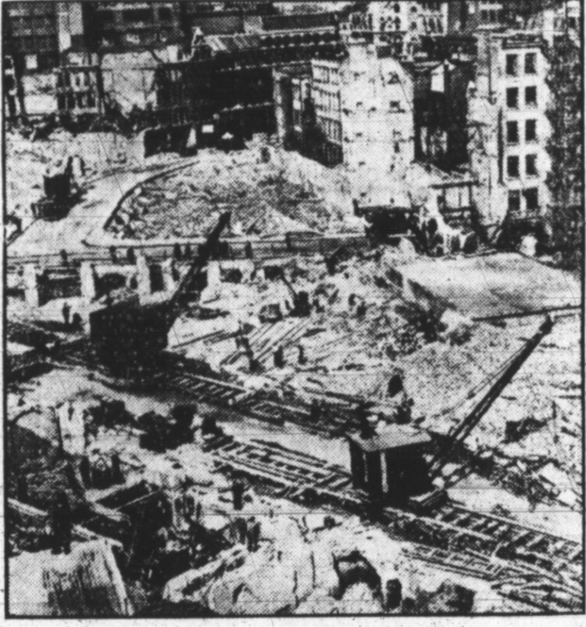
To save hundreds of thousands of tons of metal and other materials needed for her war effort, London has used the four months' lull in German air raids to clear away bomb wreckage. Four blocks of business premises demolished in the fire blitzes are being cleared here.
