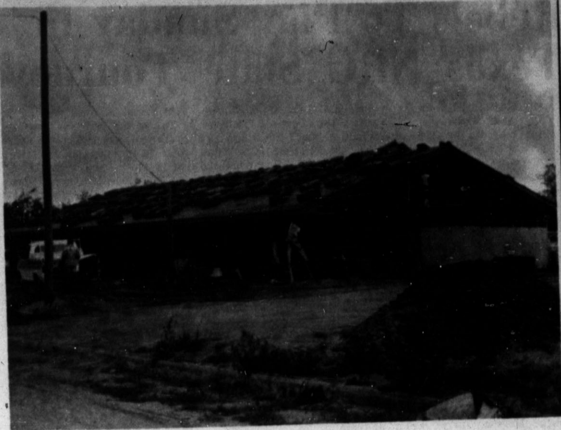
GOING UP FAST — The Campfire Girls new building is rapidly progressing, as evidenced by this photo. The building, on Fourteenth Street, is being built through contributions from the Jim Hill Estate, Hereford Lions Club, Hereford Rotary Club, and other local organizations.
